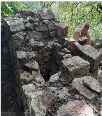
September 8 th 2022, strengthening the main structure. See Cornwall Heritage Trust FB page
